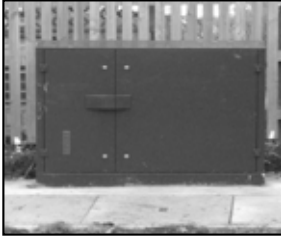
Stage 1 - Fibre Cabinet built outside the School
